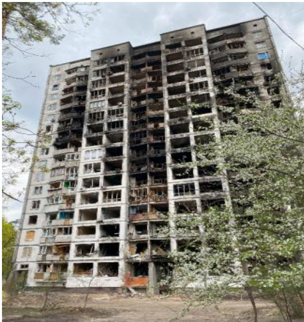
A burnt-out residential building in Kyiv after an indirect missile hit. March 15, 2022 (photo taken in April 2022). Photos of wartime Kyiv. Author: Dmytro Kolomiets
